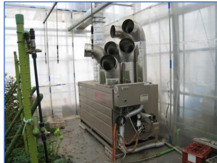
Petroleum hot air heating
