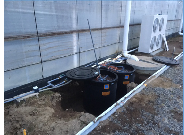
Groundwater heat exchanger
