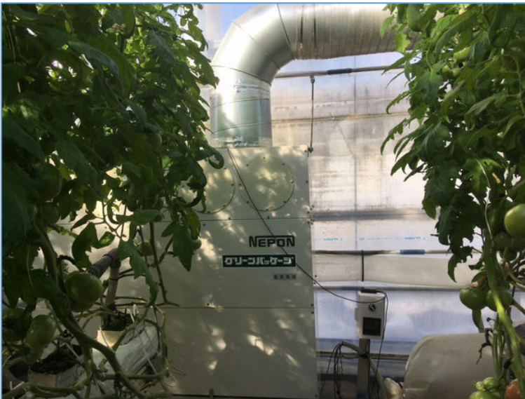
New heat pump system
